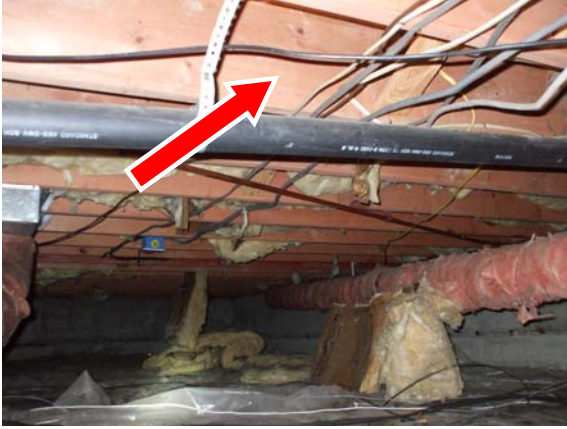
Missing under-floor insulation
