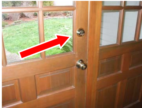
Double sided deadbolt at Front door. Key required for egress
