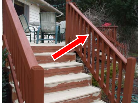
Graspable handrail missing at both stairways
