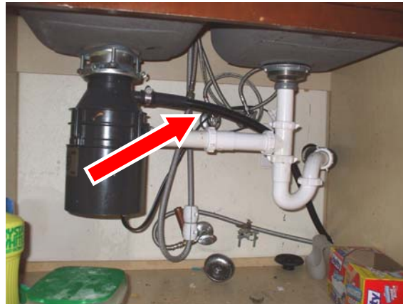
Potential cross contamination of sink drain water into dishwasher
