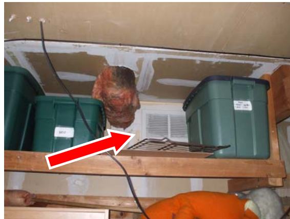
Breach of fire separation of garage to house
