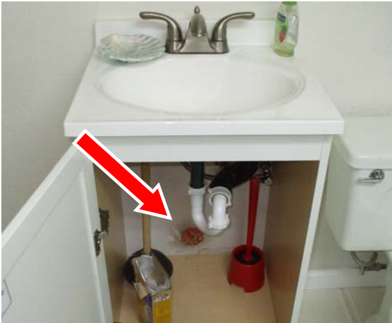
Domestic Water Shut Off
