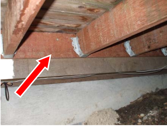
Deck ledger toe nailed to house Potential separation of deck from house
