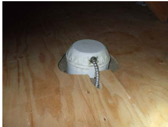
Recessed can buried in insulation and constrained by plywood
